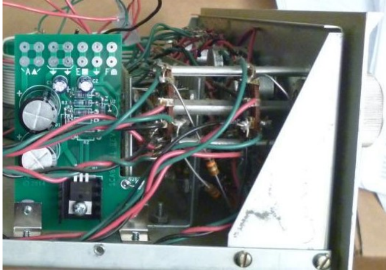
Figure 8-New Power Supply Installed in SCA80(Q)
