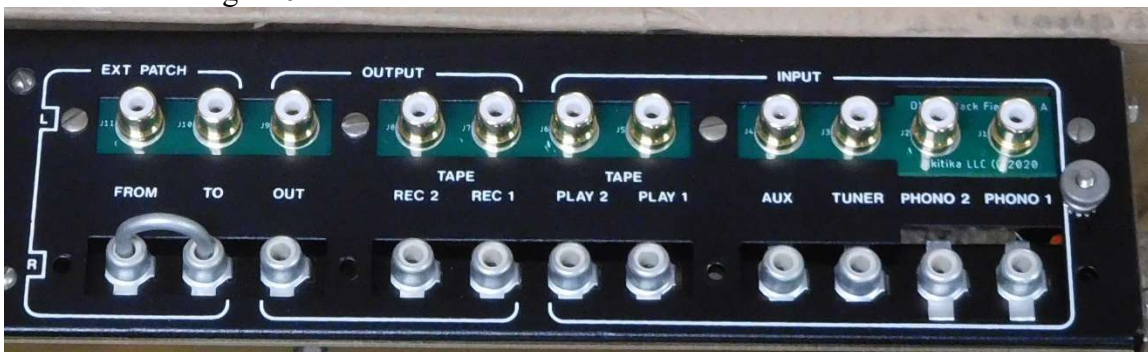
Figure 7-New left channel jack field installed
